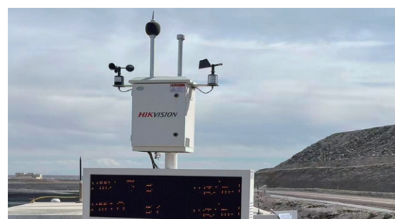
Air quality monitoring station
