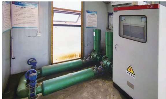
Sewage treatment facility
